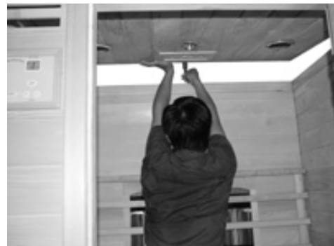
FIG-14 Leading the wires of heaters onto the board through the corresponding hole
